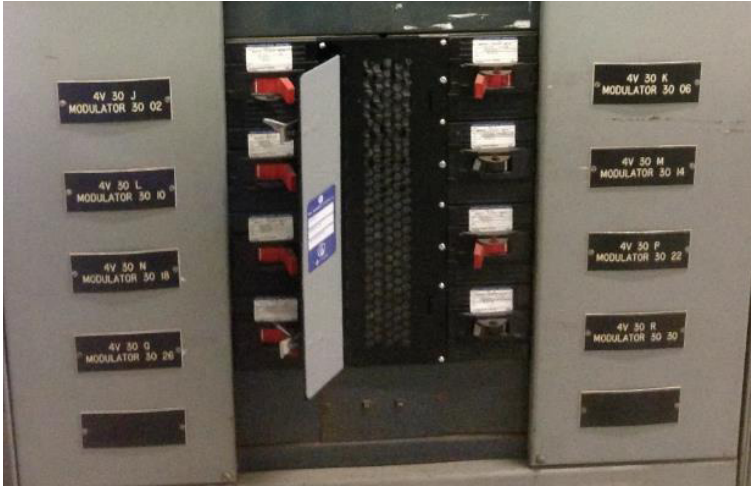
Figure 3 Custom CAP-CT window in open position for IR inspection of load side of breakers
