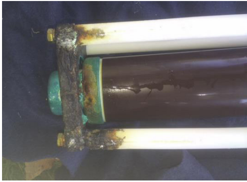
Figure 2 Evidence of water damage that would have led to the discharge activity.
