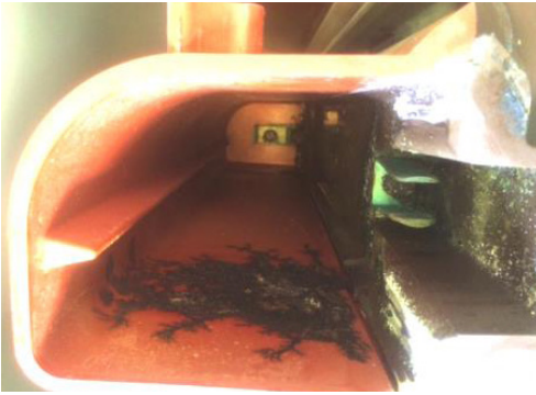
Figure 1 Extensive carbonisation on the inside surface of the fuse chamber.
